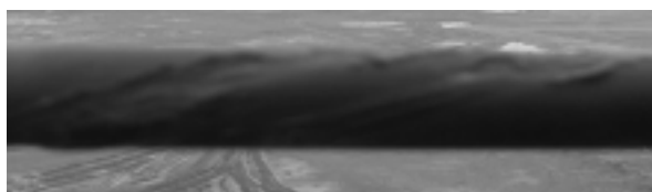
Figure 1. Helically formed corrosion tracks on the sheath of ADSS cable
